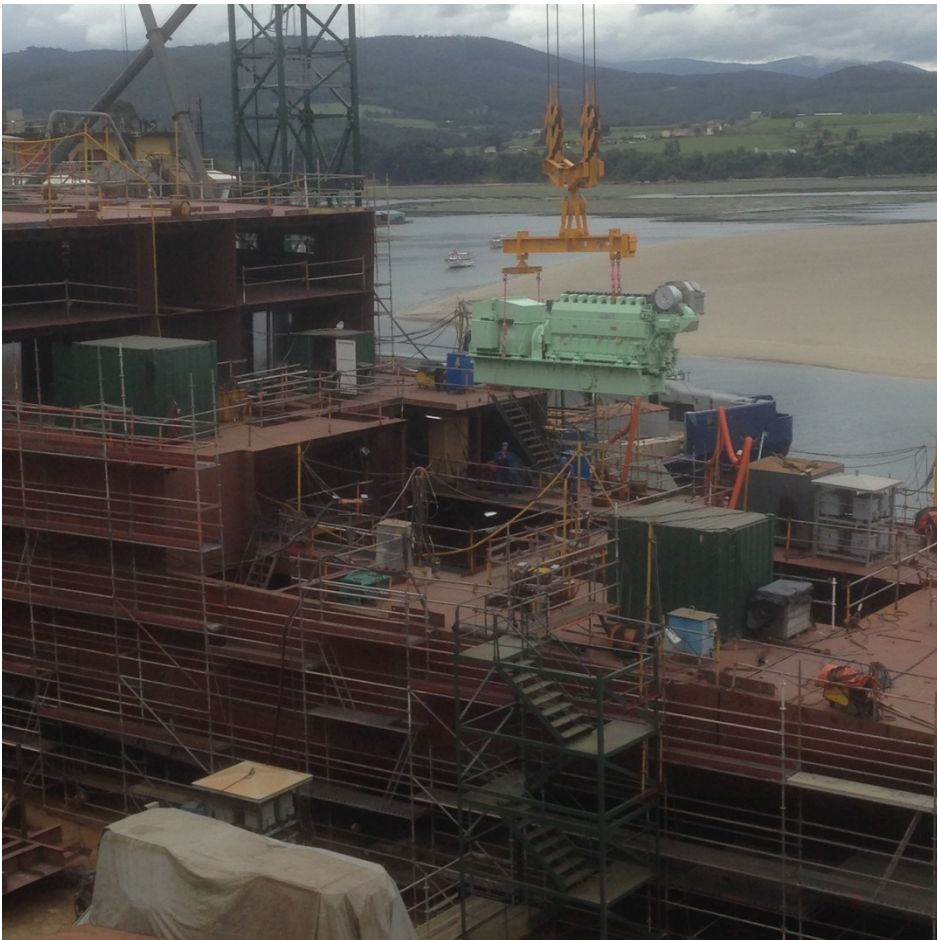
MaK Generator sets on board Sept. 3rd
