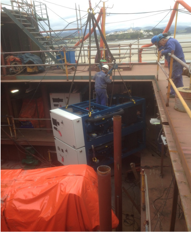
Chiller units installed in engine room
