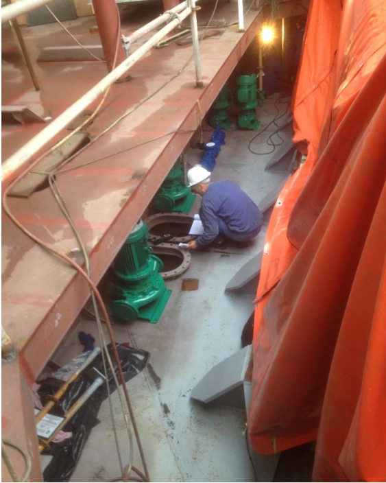
Seawater, bilge and firepumps – below T/D
