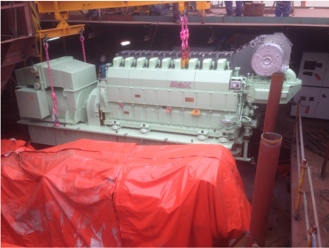
MaK Generator sets on board Sept. 3rd
