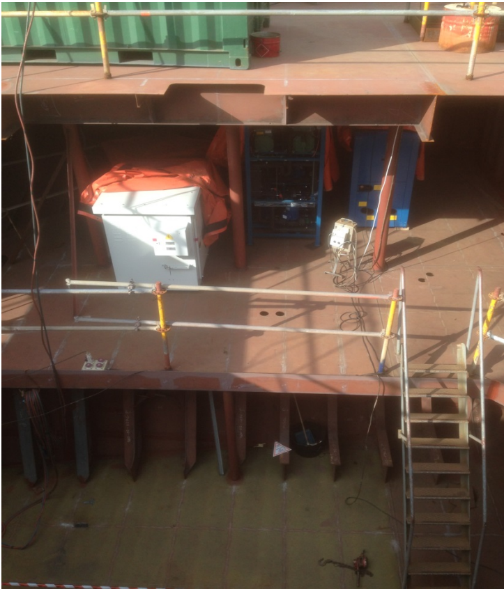
690V trafos, lab 9 cooling plant & freezer compr. in propulsion room
